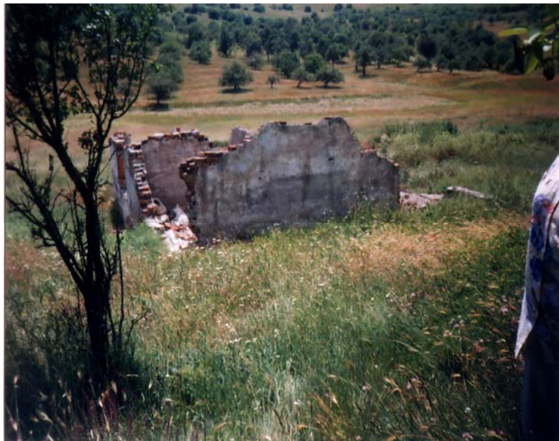
Figure 14: Warehouses for obsolete plant protection agents in bad condition
