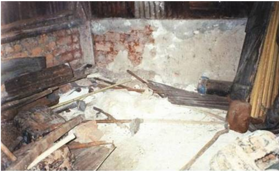
Contaminated old Pesticides store area in a Plantation section at Lugazi. Those remains may contain obsolete POPs stock and their disposal is of concern.
