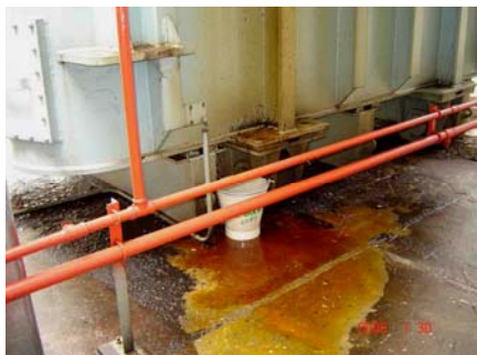
Leak from the transformer at Samanalawewa Hydro Power Station
