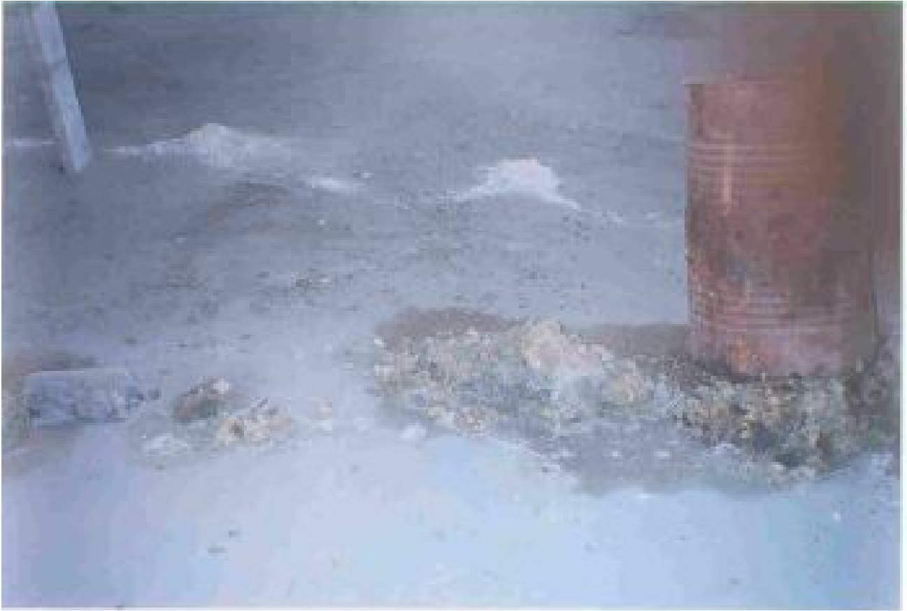
Notice leakage from the bottom of the drum (2005) Picture by Paul Maina.
