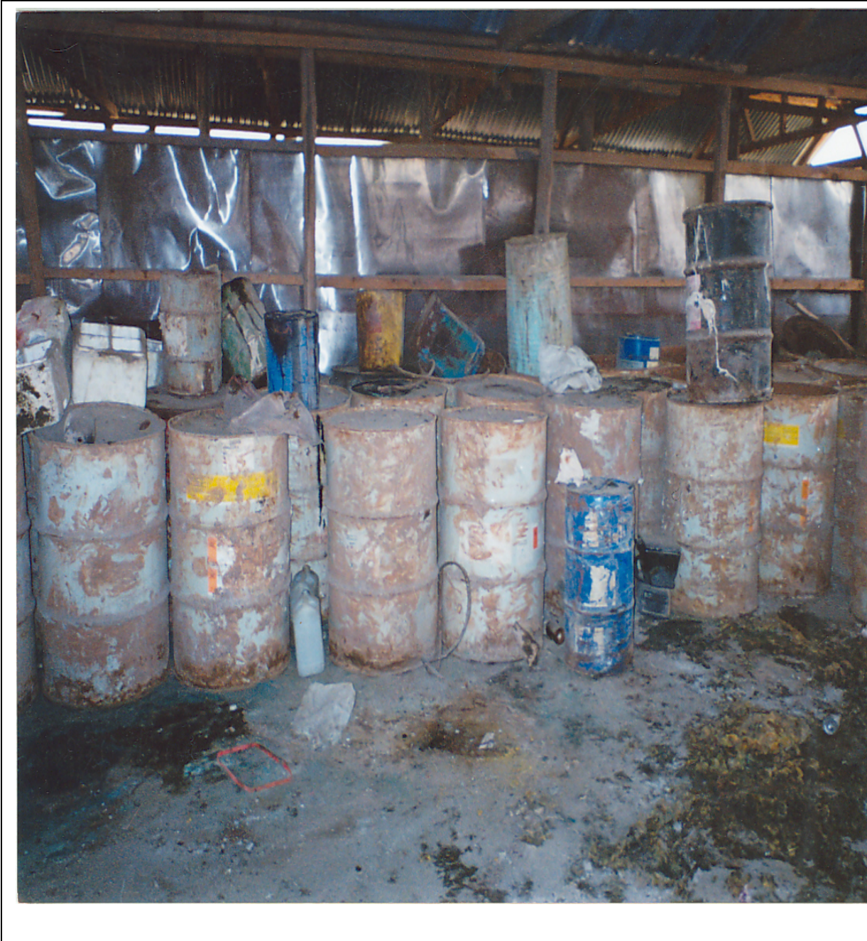
Current state of the store (2005); notice the corroded floor and chemical spillage. Picture by Rachel Wambui
