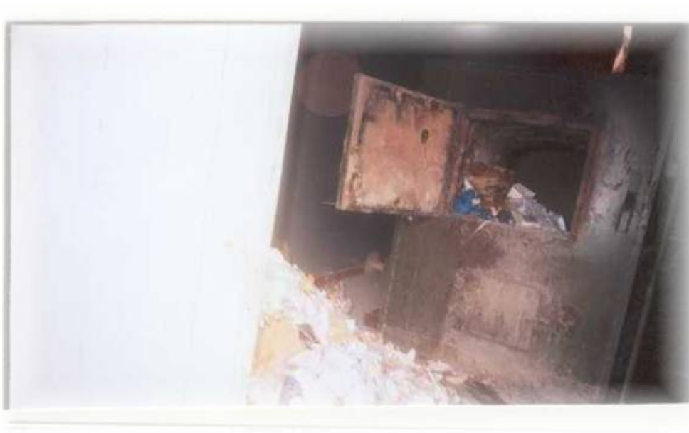
Waste burning in the incinerator
