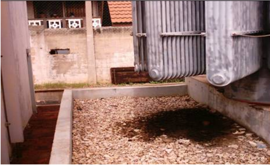
Plate 1: Immediate environ of a transformer contaminated by spillage
