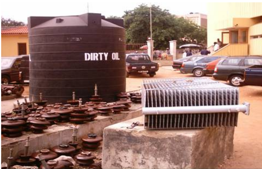
Plate 2: Displayed reservoir for PCB/oil waste at the Accra Central Power Station G
